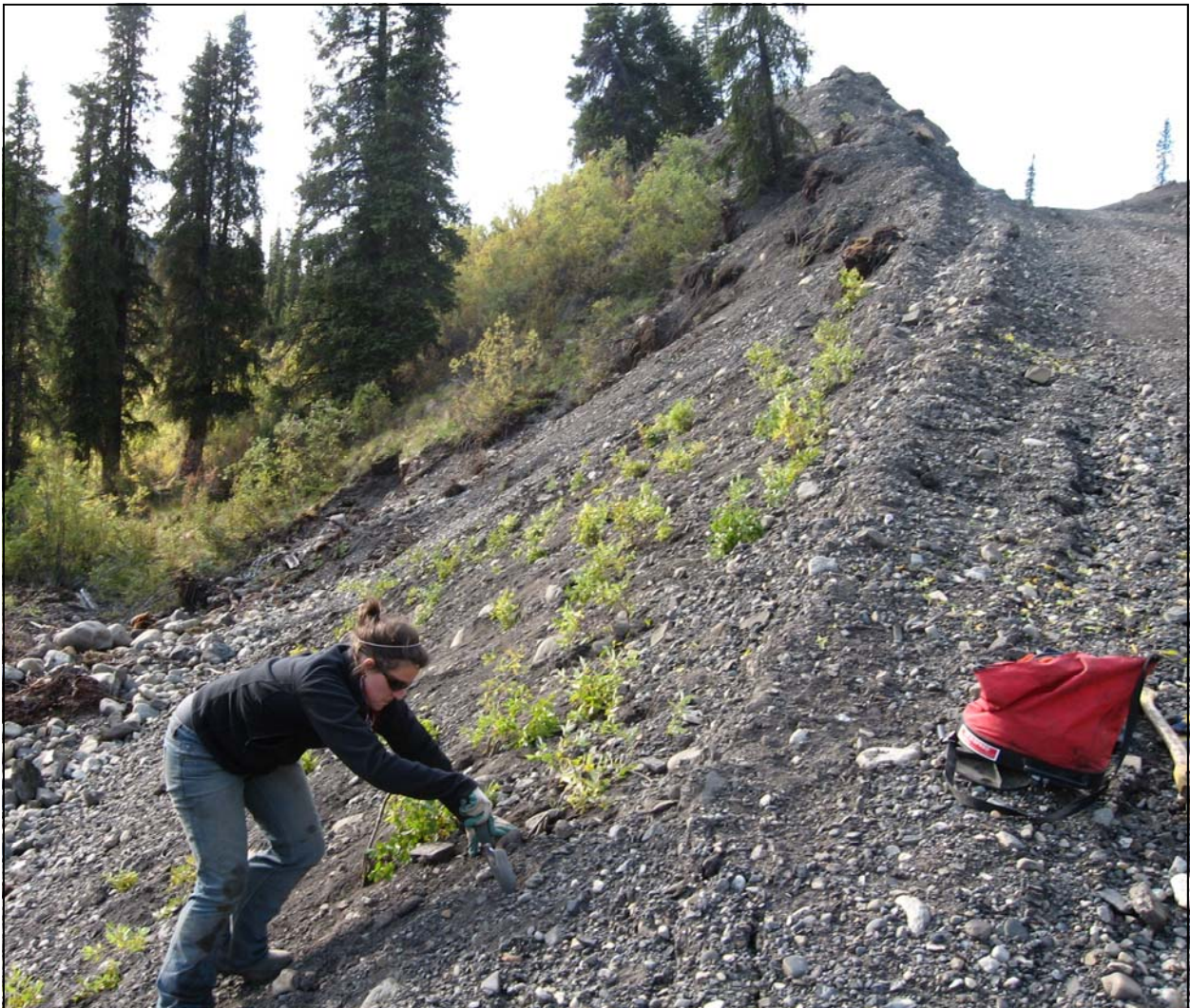
A Selwyn Resources employee reclaims a road embankment at the Selwyn Project.
